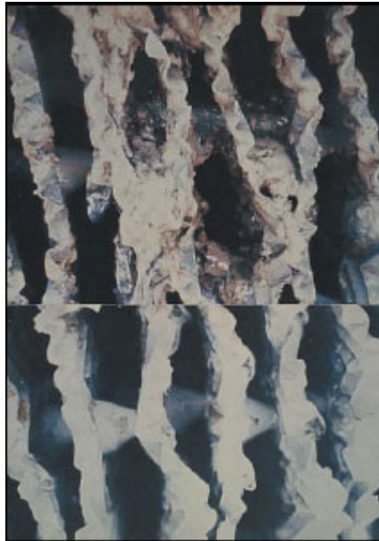
4a Composite photograph. Top--Fouled cooling tower fill. Fouling in this case was a variety of microbes and the slime they produced. Bottom--Clean cooling tower fill.
